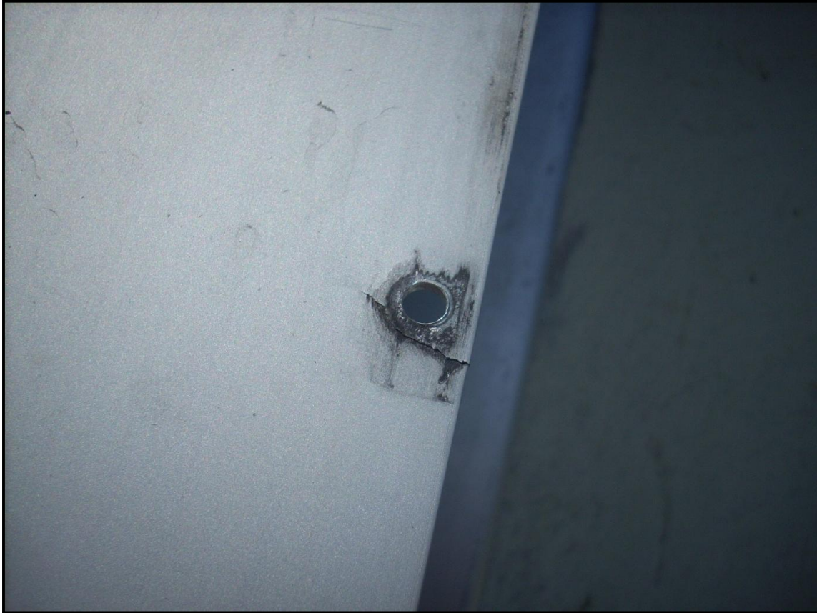
Pic.6. Example of crack – it makes mast change mandatory
